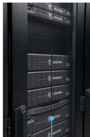
Rack sensors ensure the correct amount of cold air is provided to eliminate hot spots.
